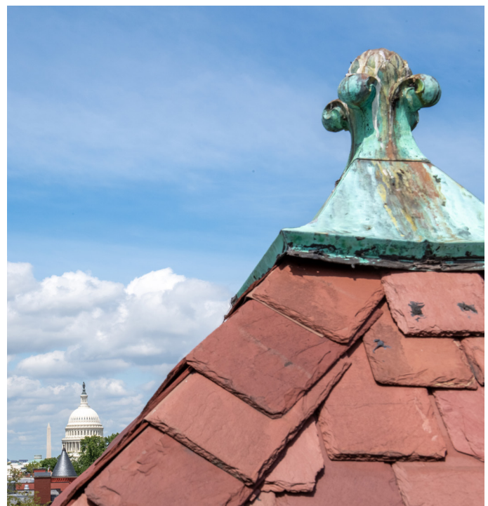
The finial on the roof of Friends Place on Capitol Hill is in the foreground, with the Capitol and Washington Monument nearby.
